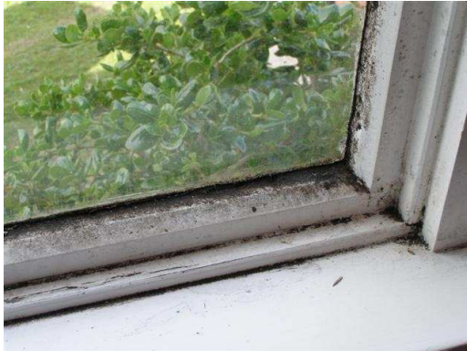
2. Mould on window in bedroom
