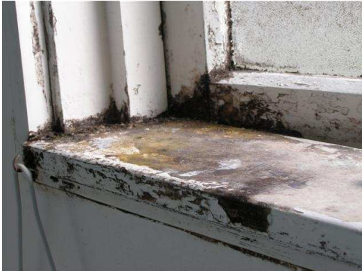
1. Mould on window sill in bathroom
