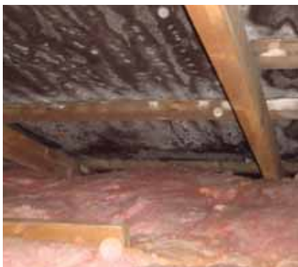
Figure 1: Moisture is clearly visible on the roofing underlay.
